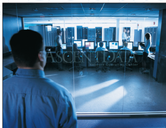
Network Operations Center (NOC)
